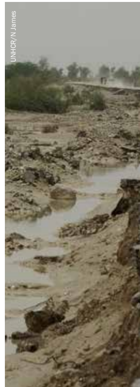
Road damaged by floods in Balochistan, Pakistan, 2010.
